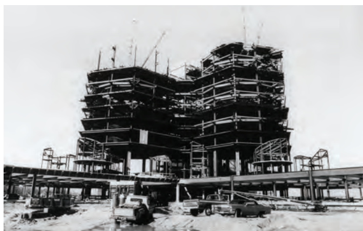
University Hospital under construction in the late 1970s. See Pages 12-13 for picture of it now, plus our history.
